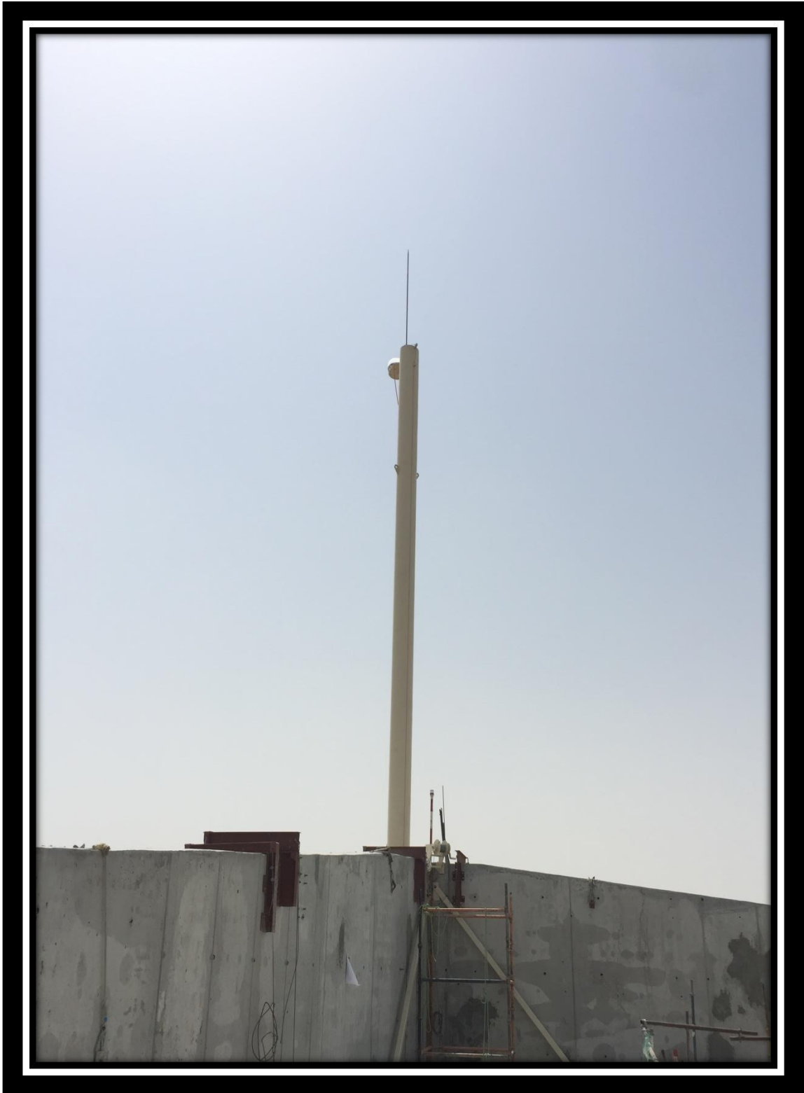
Roof High Mast Installed
